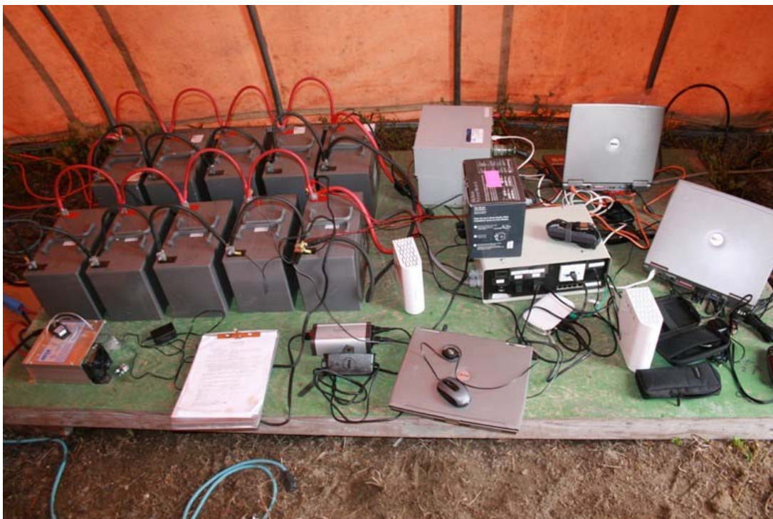
Photo 3. Control box, NAS and power source for the Site 1 sonar system housed in the WeatherPort tent, 2009.
